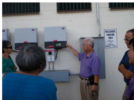
Richard explains about the Inverters.
